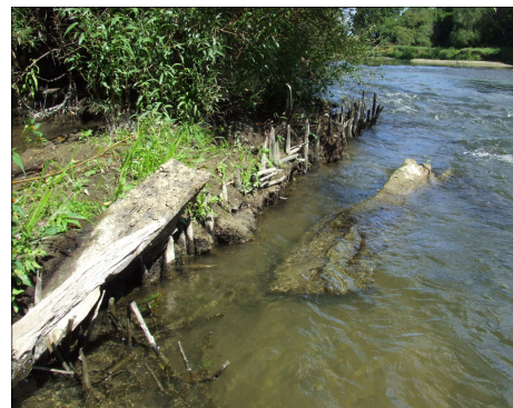
The eel weir remains, photographed by Tony Roxburgh. The line of posts runs parallel to the river flow.
