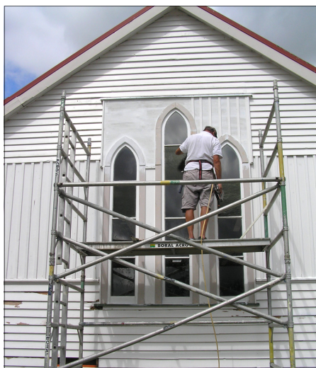
Maintenance under way on the west windows. The newly-installed flashing can be seen above the windows.
